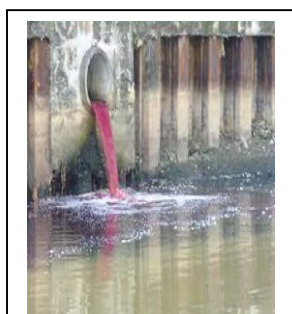
Discharge of sullage directly into drainage system
